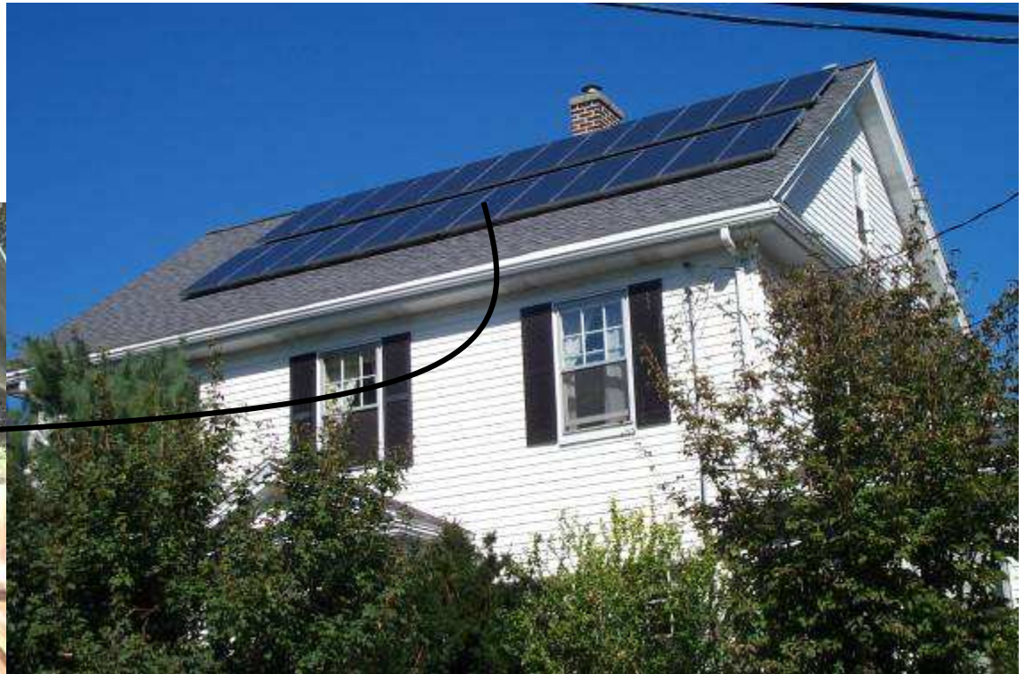
Residential PV Installation – Boston 24 Evergreen Solar EC-100 modules
