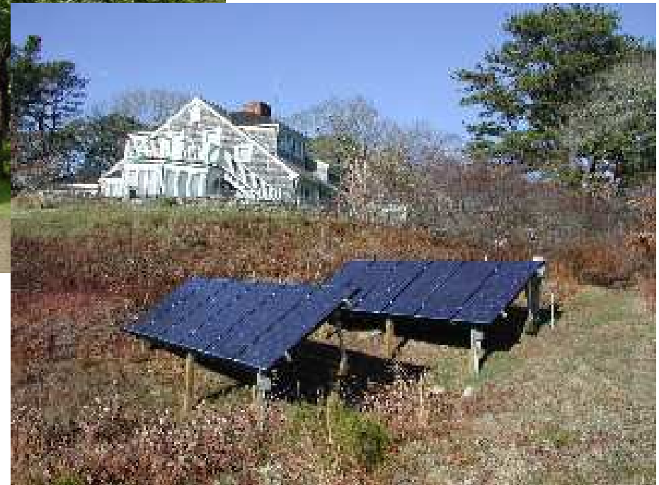
Wendell, MA pole-mounted system installed by PV Squared August 2003
