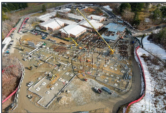
West Elementary and Shawsheen Preschool: Steel framing is being erected in the foreground. West Elementary school is visible at the rear of this photo.
