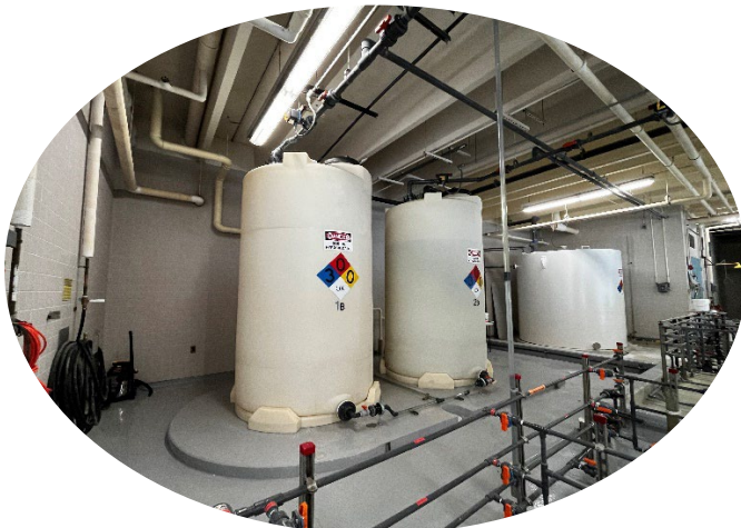
Two new sodium hypochlorite storage tanks
