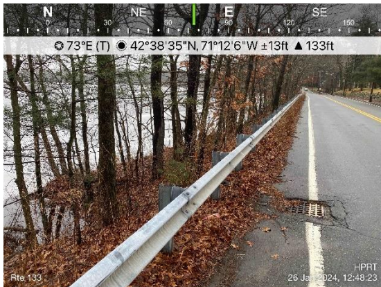
Figure 6. Direct discharge of untreated Route 133 stormwater.
