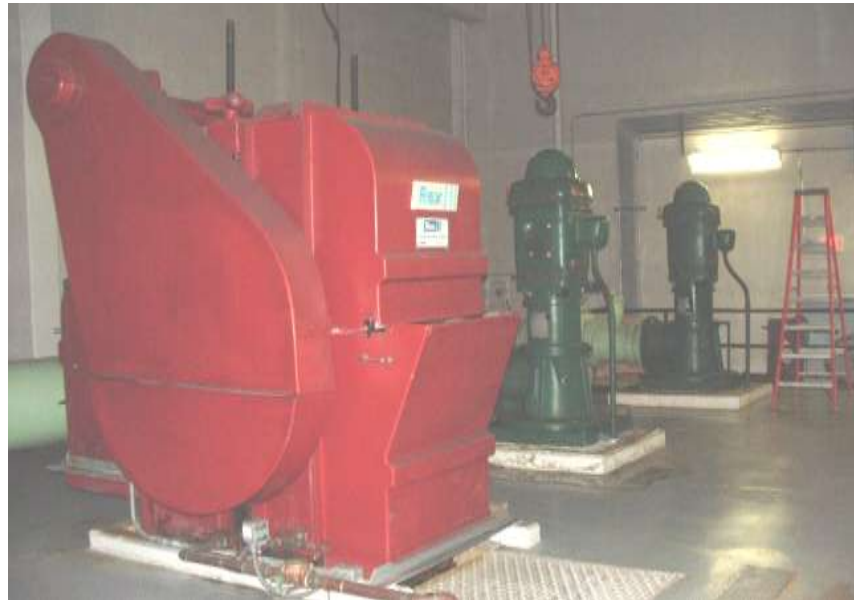
This photo shows the screen (the red structure on the left) and the raw water pumps in the background.
