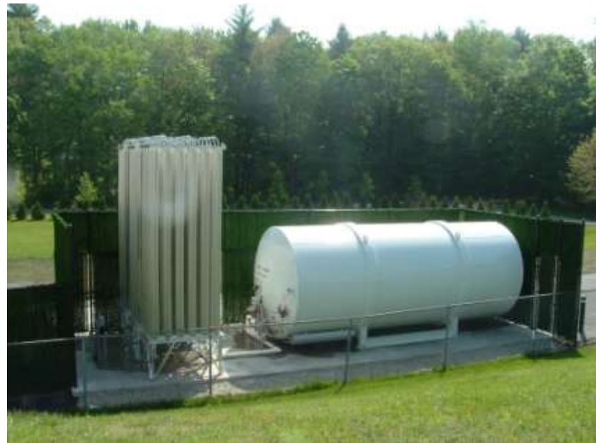
Liquid oxygen storage tank and vaporizers.
