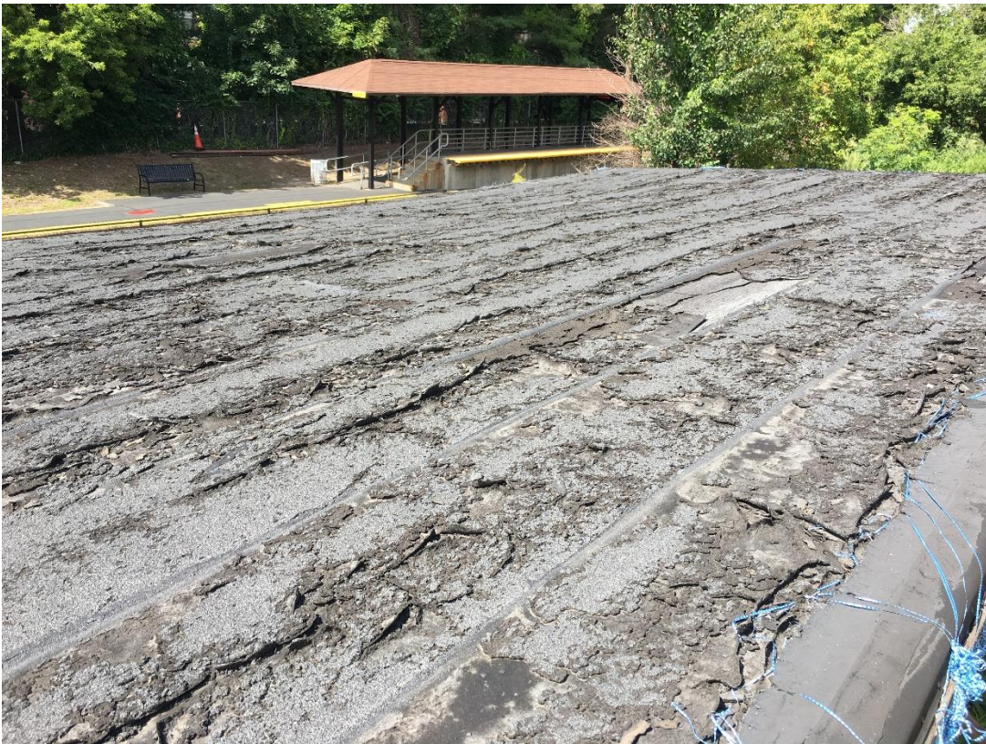
A representative view of the asbestos-containing roof material on the shed
